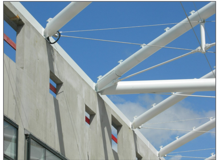
Tension-only elements in real project: Coverage of the atrium, Helios Building; Baudin Châteauneuf
